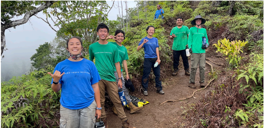
KUPU interns take a break from repairing the stairs at the top of Kuli'ou'ou Ridge Trail.
